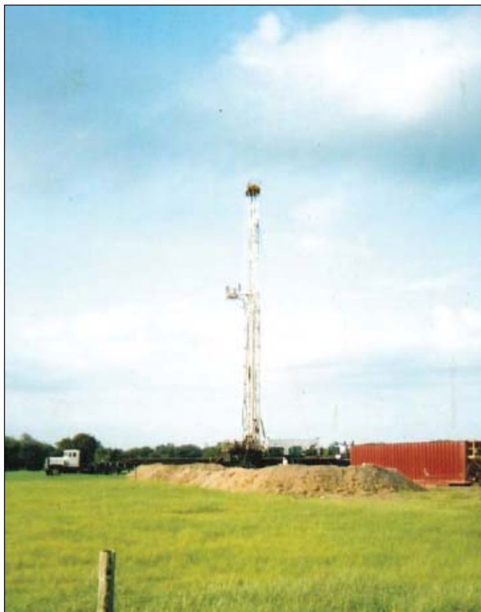
Titan Drilling Co.'s Rig No. 3 is drilling 10 wells for Magnus Oil & Gas Corp. in a new gas field in Goliad County, Tex. (photo from Magnus; Fig. 1).
